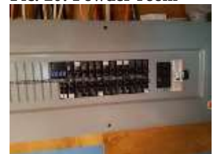
Pic. 24: 200 amp breaker panel with all copper wire
