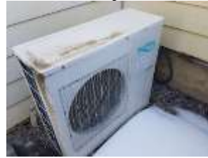
Pic. 7: AC unit
