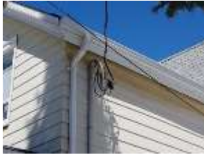
Pic. 5: Service drop
