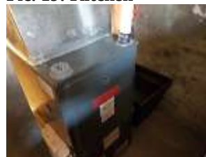
Pic. 23: High efficiency gas furnace
