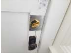
Pic. 9: Key lock needed for rear platform door – no railing on platform
