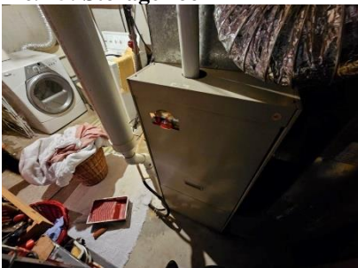
Pic. 28: Gas furnace 1990
