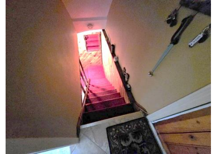
Pic. 21: Handrailing advised for basement stairwell
