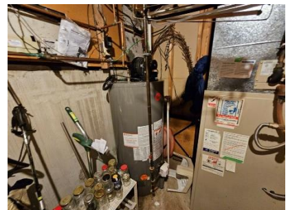
Pic. 27: Rental hot water tank
