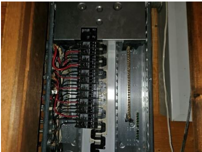
Pic. 22: 100 amp main breaker panel – mix of aluminum and copper wire
