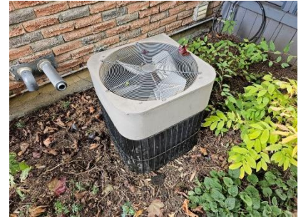
Pic. 3: AC unit 1989
