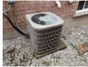
Pic. 3: AC unit
