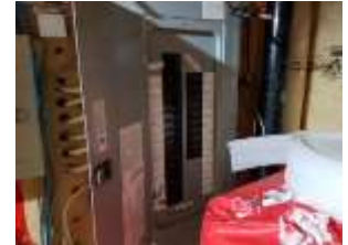
Pic. 28: 100 amp breaker panel, all copper wire
