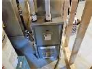
Pic. 26: High efficiency gas furnace
