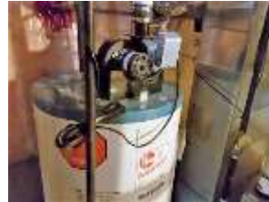
Pic. 27: Rental hot water tank
