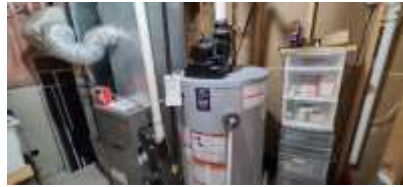
29: Rental hot water tank 2021
