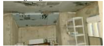
33: Polystyrene insulation in cold room
