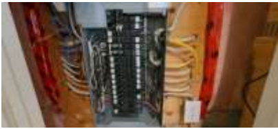
34: 100 amp breaker panel
