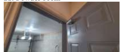
24: No auto closer on garage entry door
