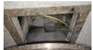
Pic. 20: Fireplace not functional being converted to gas
