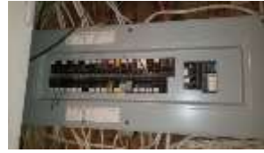
Pic. 35: 200 amp breaker panel with all copper wire
