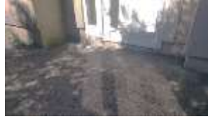
Pic. 3: Low grading at side entrance
