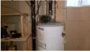
Pic. 33: Rental hot water tank
