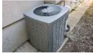
Pic. 7: AC unit 2018
