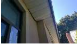
Pic. 6: Soffit section in need of repair
