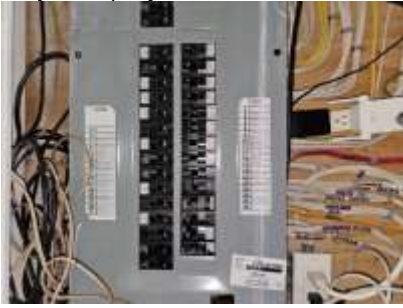
Pic. 31: 100 amp breaker panel
