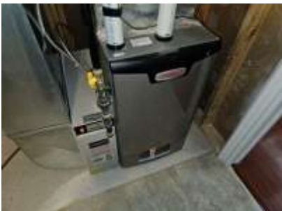
Pic. 28: Gas furnace 2015
