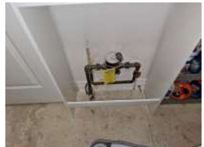
Pic. 30: Water main
