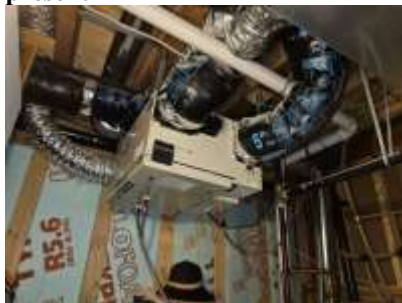
Pic. 29: HRV system
