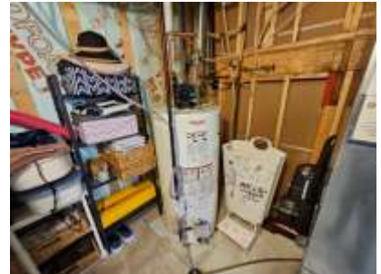
Pic. 27: Hot water tank present
