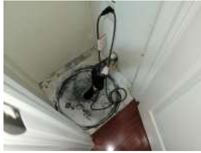
Pic. 32: Sump pump
