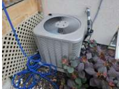
Pic. 5: AC unit 2015
