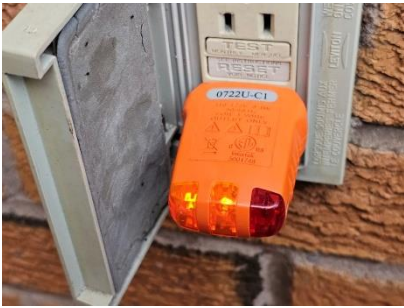
Pic. 4: Exterior GFCI won't trip
