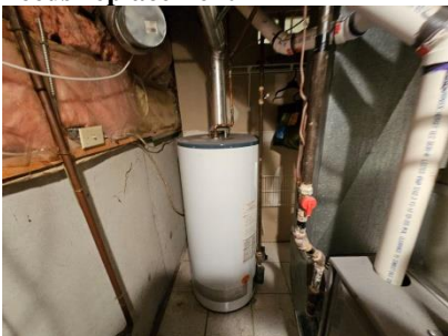
Pic. 28: Hot water tank 2009
