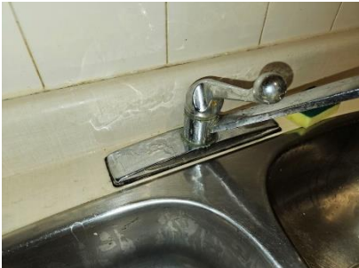
Pic. 25: Sink faucet broken and needs replacement
