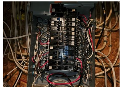
Pic. 30: 100 amp breaker panel
