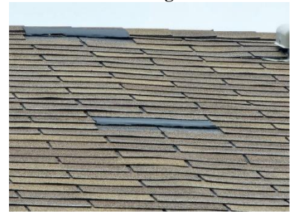
Pic. 6: Missing shingle tab on rear roof
