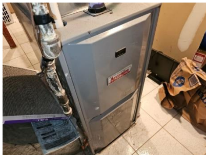
Pic. 29: Gas furnace 2010
