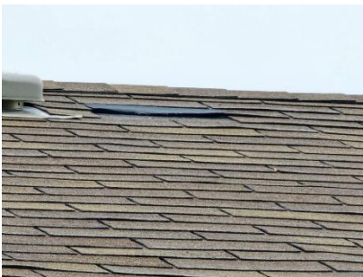
Pic. 7: Missing shingle tab on rear roof
