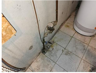
Pic. 32: Water main
