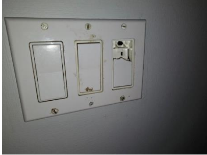
Pic. 34: Broken light switch on rec room
