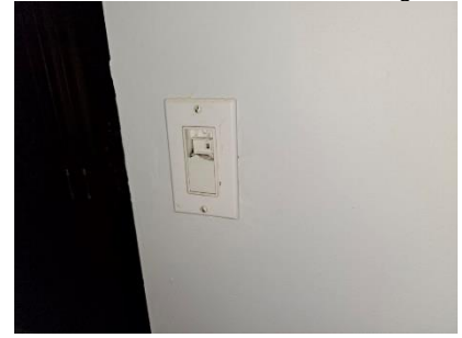
Pic. 33: Broken light switch on rec room
