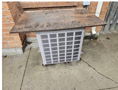
Pic. 8: AC unit 2011
