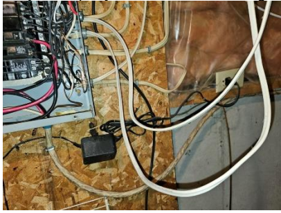
Pic. 31: Loose wires should be properly secured
