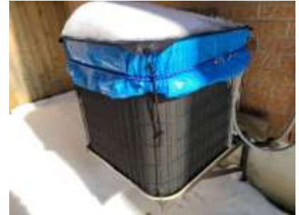
Pic. 3: AC unit
