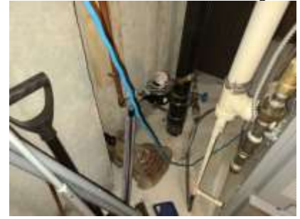
Pic. 33: Water main
