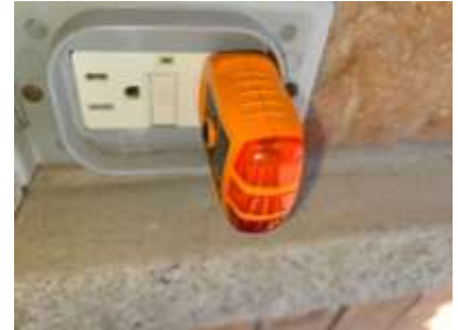
Pic. 6: Front GFCI outlet no power
