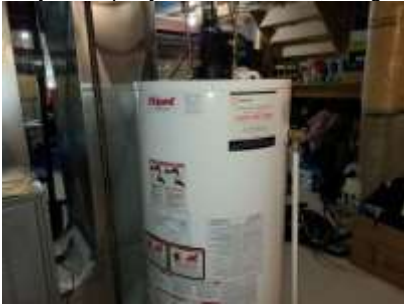
Pic. 31: Rental hot water tank
