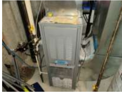
Pic. 32: Gas furnace
