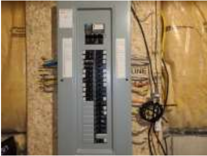
Pic. 34: 200 amp breaker panel
