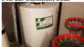
Pic. 26: Hot water tank
