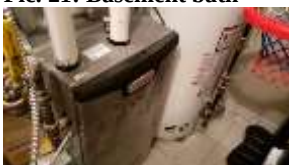
Pic. 25: Gas furnace 2014
