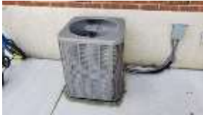
Pic. 5: AC unit 2014
