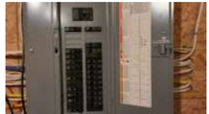
Pic. 27: 100 amp breaker panel
