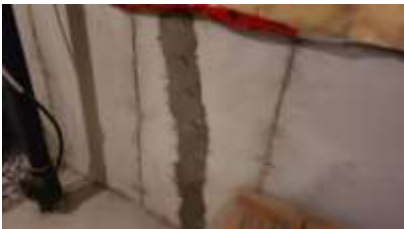
Pic. 25: Professionally repaired foundation crack
