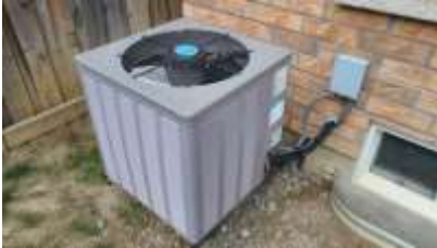
Pic. 4: AC unit
