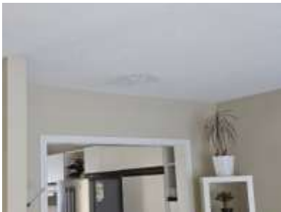
Pic. 37: Old water damage on living room ceiling - repaired
