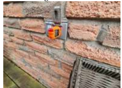
Pic. 9: No power at rear outlet and light
