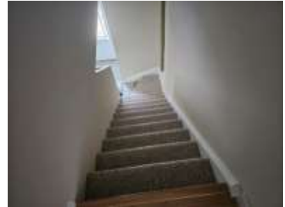
Pic. 21: Main stairwell, recommend adding a full handrailing
