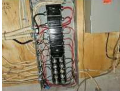
Pic. 35: 100 amp fuse panel
