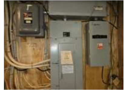
Pic. 36: 200 amp main service wires
