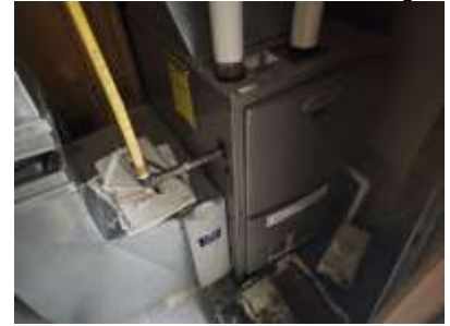
Pic. 33: Gas furnace 2017
