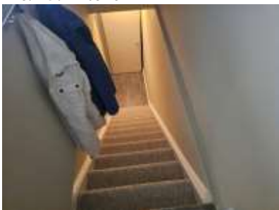
Pic. 28: Handrailing advised for basement stairwell
