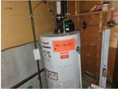
Pic. 34: Rental hot water tank 2011
