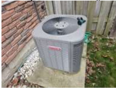
Pic. 5: AC unit 2017
