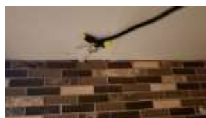
Pic. 26: Open air junction for under cabinet lights – wiring joint should be in a junction box
