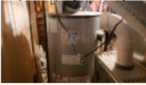
Pic. 33: Owned hot water tank
