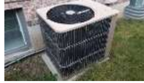
Pic. 3: AC unit 1998
