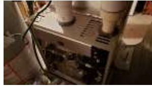
Pic. 34: Gas furnace 2012
