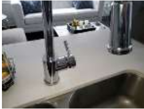
Pic. 25: Loose faucet
