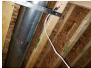
Pic. 30: Loose wire in rough in bathroom
