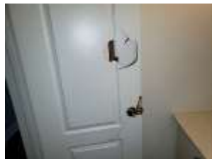
Pic. 18: Damaged bathroom door
