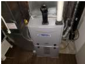
Pic. 33: Gas furnace
