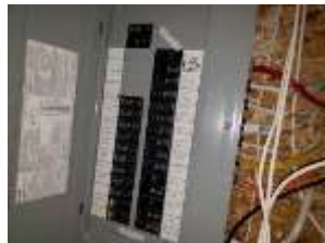
Pic. 34: 100 amp breaker panel
