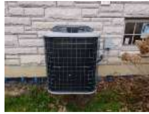
Pic. 3: AC unit
