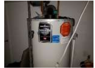
Pic. 32: Rental hot water tank
