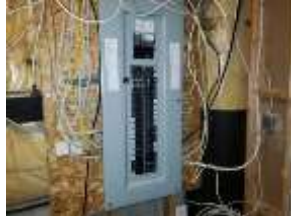
Pic. 42: 200 amp breaker panel
