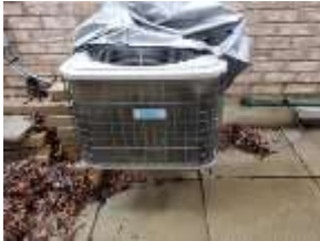
Pic. 5: AC unit
