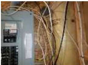
Pic. 45: Loose wires around panel should be secured
