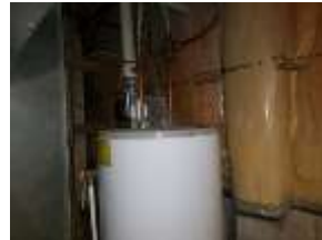
Pic. 39: Hot water tank
