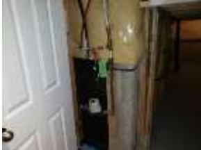
Pic. 41: Water main
