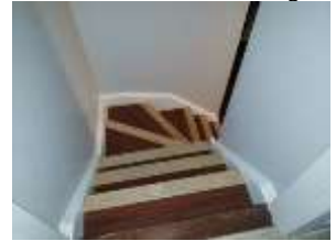
Pic. 32: Handrailing needed for basement stairwell
