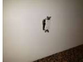
Pic. 35: Loose outlet needs to be secured
