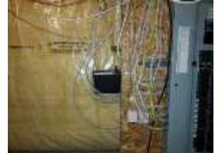
Pic. 44: Loose wires around panel should be secured
