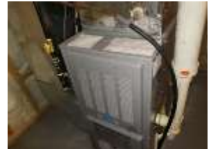
Pic. 40: Gas furnace
