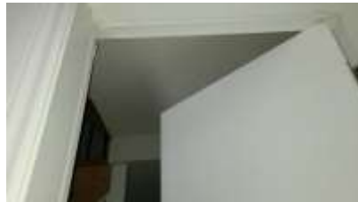
Pic. 8: Auto closer needed for garage entry door for safety
