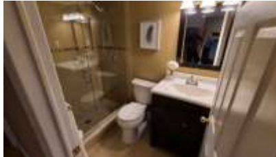
Pic. 23: Basement bath – outlet needs to be GFCI protected
