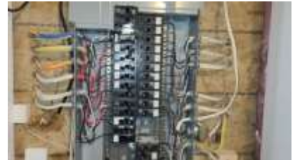
Pic. 27: 100 amp breaker panel with all copper wire
