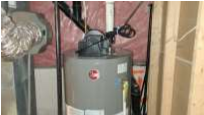
Pic. 25: New rental hot water tank
