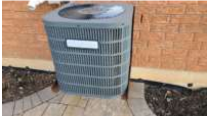
Pic. 4: AC unit 2005
