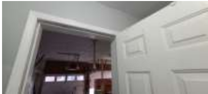
Pic. 7: Auto close needed for garage entry door
