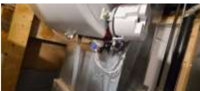
Pic. 37: Humidifier leaking
