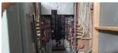
Pic. 38: 100-amp breaker panel
