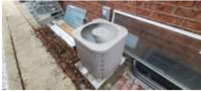
Pic. 4: AC unit 2002
