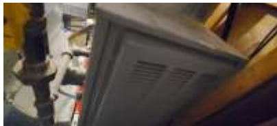
Pic. 35: Gas furnace 2002
