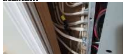
Pic 38: Open air wiring junction needs to be corrected
