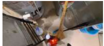
Pic. 36: Water on floor from humidifier
