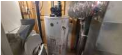
Pic. 34: Hot water tank 2012
