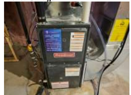
Pic. 9: Gas furnace 2022
