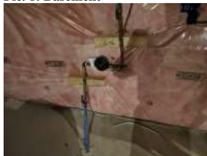
Pic. 11: Water main
