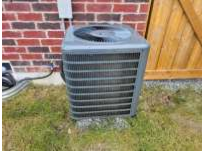
Pic. 4: AC unit 2021
