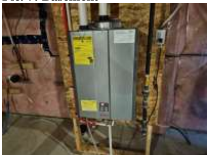
Pic. 10: Tankless hot water system 2022
