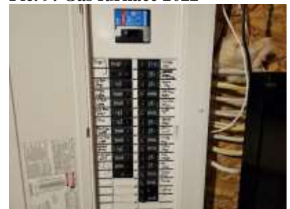
Pic. 12: 200 amp breaker panel
