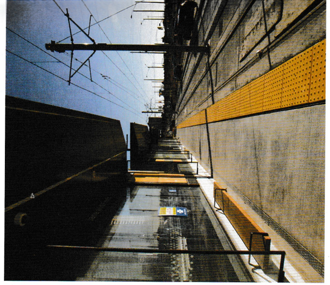
Photo: The high voltage overhead catenary system on the guideway at the Jane and Finch stop.
