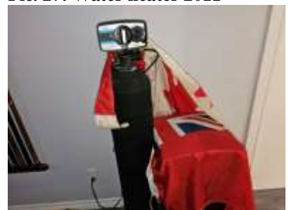
Pic. 30: Water softener
