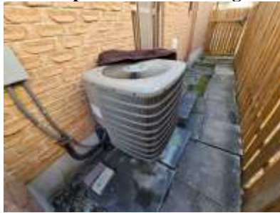
Pic. 5: AC unit 2015
