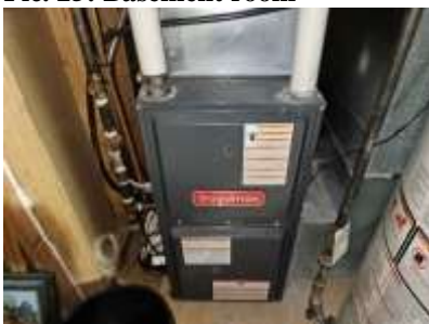
Pic. 28: Gas furnace 2015
