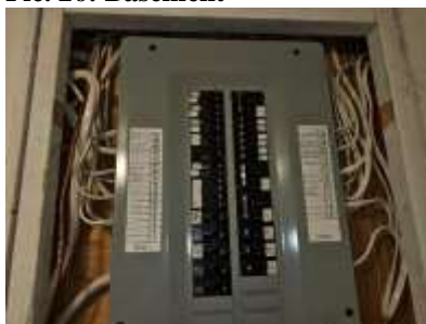
Pic. 29: 100 amp breaker panel
