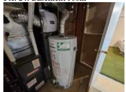
Pic. 27: Water heater 2011
