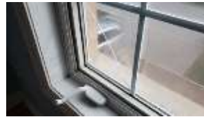
Pic. 15: Cracked window panel
