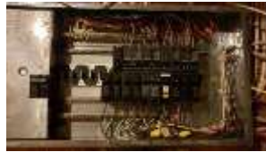
Pic. 34: 100 amp breaker panel
