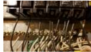
Pic. 35: Double tapped breaker
