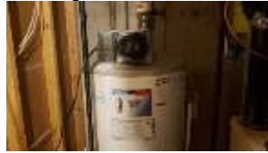
Pic. 30: Rental hot water tank
