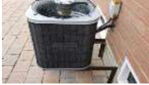
Pic. 5: AC unit
