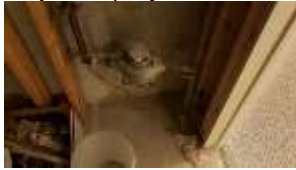
Pic. 29: Water main
