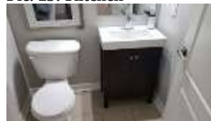
Pic. 27: Powder room – water to toilet shut off and could not be tested
