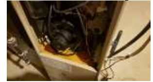
Pic. 32: Past water damage and some rusting inside
