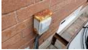
Pic. 6: AC disconnected needs to be properly secured to the wall
