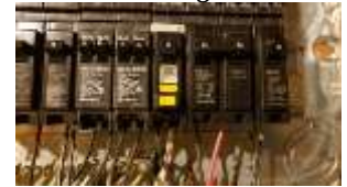
Pic. 36: ARCF breaker defective and should be replaced
