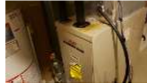
Pic. 31: Gas furnace
