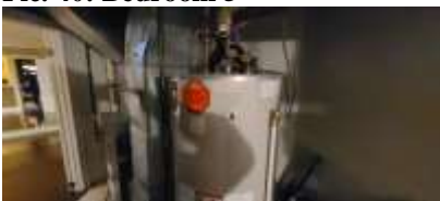
Pic. 43: Water heater 2011
