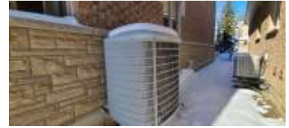
Pic. 3: AC unit 2008
