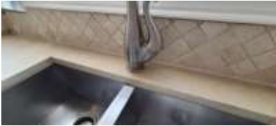
Pic. 31: Sink faucet loose
