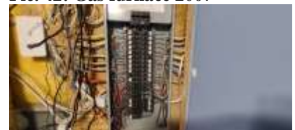
Pic. 45: 200 amp breaker panel
