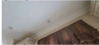
Pic. 32: Pot light over sink defective
