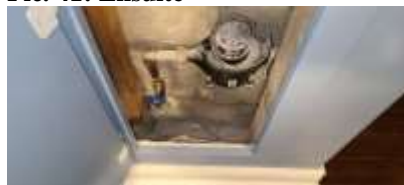
Pic. 44: Water main
