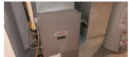
Pic. 42: Gas furnace 2007
