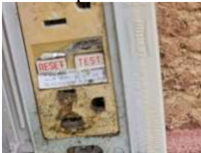
Pic. 7: Lower half of rear GFI plugged up
