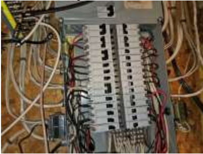
Pic. 37: 100 amp breaker panel
