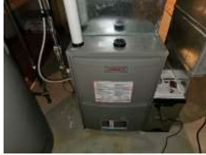
Pic. 35: Gas furnace 2019
