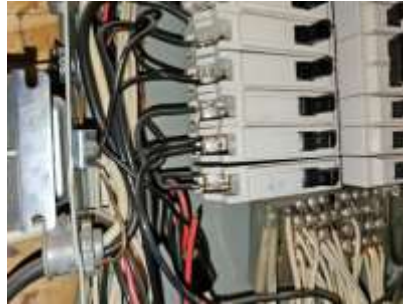
Pic. 38: 2 breaker double tapped
