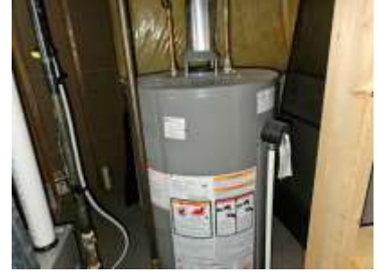
Pic. 36: Water heater 2013
