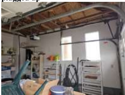
Pic. 10: Garage – south safety sensors not aligned
