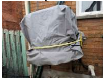
Pic. 8: AC unit 2019
