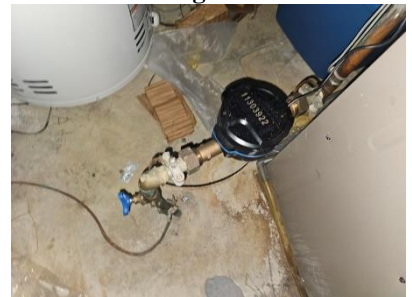
Pic. 39: Water main
