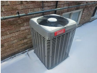
Pic. 7: AC compressor 2020
