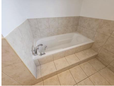
Pic. 20: 2 nd floor bathroom
