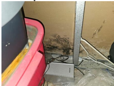
Pic. 38: Visible apparent mould growth in furnace room
