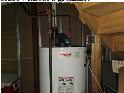
Pic. 40: Water heater 2020
