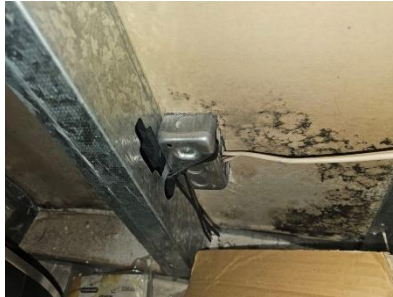
Pic. 35: Outlet box wired incorrectly
