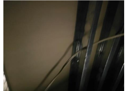
Pic. 36: Romex run thru metal studs without a grommet
