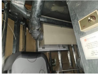
Pic. 47: HRV system
