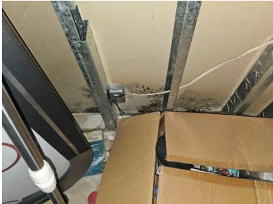
Pic. 34: Visible apparent mould growth in furnace room
