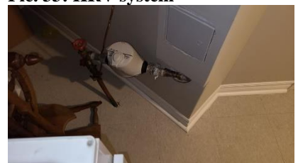
Pic. 36: Water main
