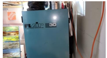
Pic. 33: HRV system
