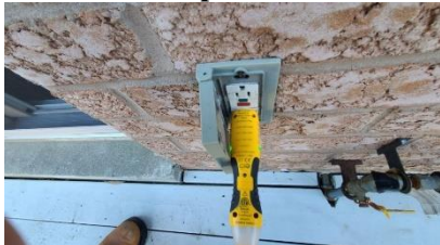
Pic. 7: Rear GFCI outlet defective – won't trip and should be replaced
