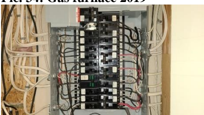
Pic. 37: 100 amp breaker panel
