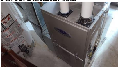
Pic. 34: Gas furnace 2019
