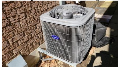
Pic. 5: AC unit 2019
