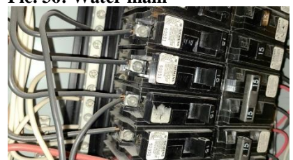
Pic. 39: Double tapped breaker
