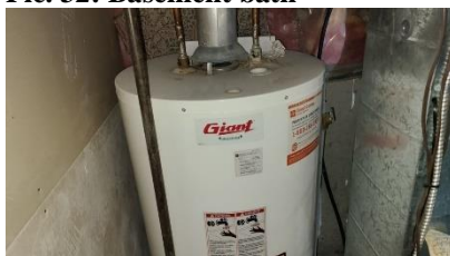
Pic. 35: Hot water tank 2014
