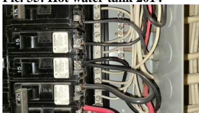
Pic. 38: Double tapped breaker
