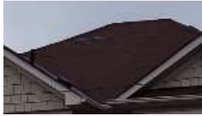
Pic. 2: Missing shingle tabs at the front of the house
