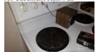
Pic. 32: Back left stove burner not working
