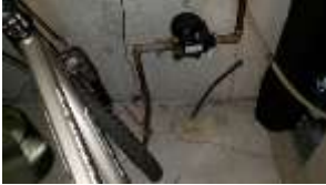
Pic. 37: Water main
