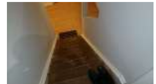
Pic. 28: Handrailing need for basement stairwell
