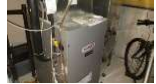
Pic. 36: Gas service
