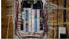
Pic. 38: 100 amp breaker panel
