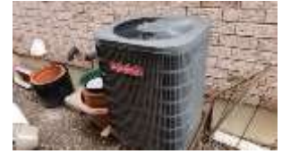
Pic. 4: AC unit
