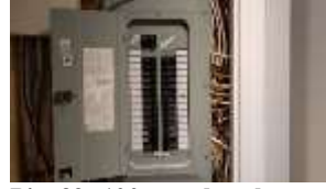
Pic. 39: 100 amp breaker panel
