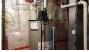
Pic. 37: New hot water tank – rental
