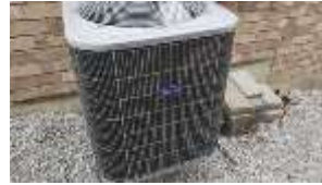
Pic. 3: AC unit
