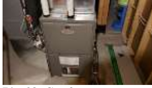
Pic. 38: Gas furnace
