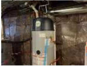
Pic. 25: Hot water / boiler system
