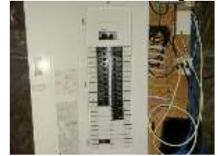
Pic. 28: 200 amp main electrical panel with all copper wire
