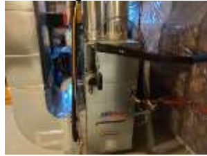
Pic. 26: Hot water / fan coil furnace
