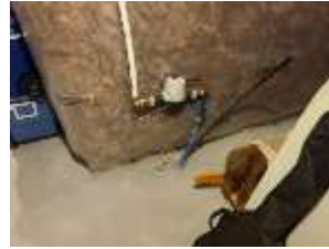
Pic. 27: Water main
