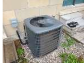
Pic. 3: AC unit
