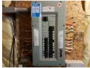
Pic. 30: 100 amp breaker panel – all copper wire
