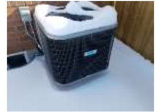
Pic. 4: AC unit
