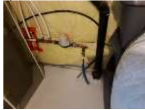
Pic. 26: Water main
