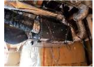
Pic. 28: HRV system
