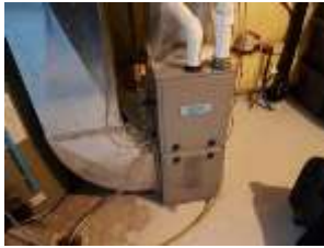
Pic. 29: High efficiency gas furnace
