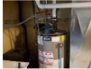
Pic. 27: Rental hot water tank
