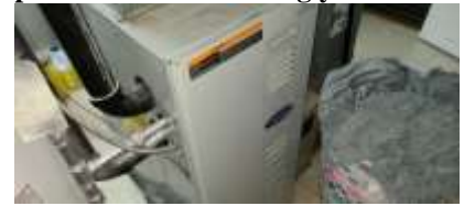
Pic. 33: Gas furnace 2000
