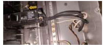
Pic. 36: 1 breaker double tapped
