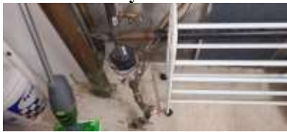
Pic. 34: Water main
