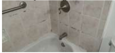
Pic. 29: Typical mould / mildew present clean accordingly
