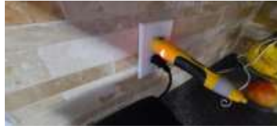
Pic. 23: Outlet to the right of the sink is not wired correctly
