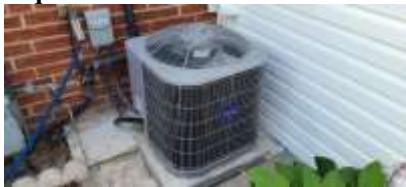
Pic. 7: AC unit 2020
