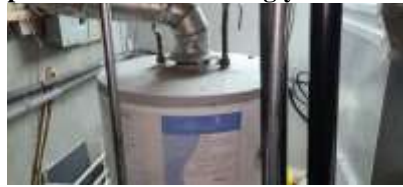
Pic. 32: Rental hot water tank 2009
