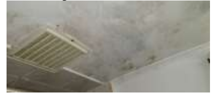
Pic. 30: Typical mould / mildew present clean accordingly
