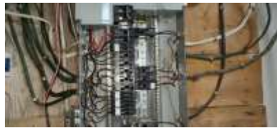
Pic. 35: 100 amp breaker panel
