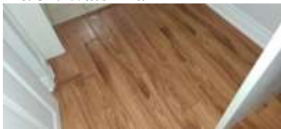
Pic. 37: Old water damage to flooring outside basement eating area
