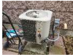
Pic. 3: Original AC unit
