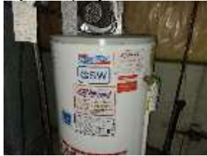
Pic. 25: Rental hot water tank
