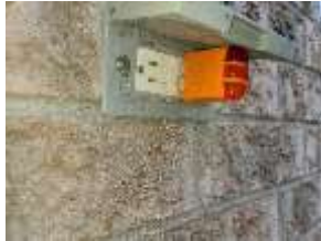
Pic. 5: Rear GFCI outlet defective and needs to be replaced
