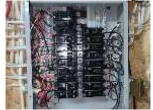
Pic. 28: 100 amp breaker panel
