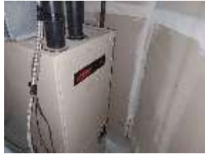
Pic. 26: Original gas furnace
