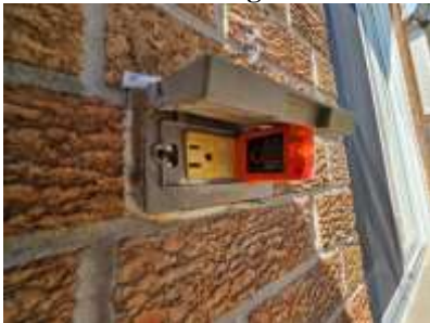
Pic. 7: Rear GFCI outlet will not trip and should be replaced
