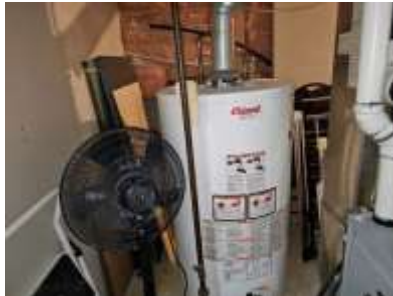
Pic. 38: Hot water tank 2020
