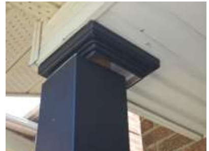
Pic. 9: Support post cover separated at soffit, repair accordingly
