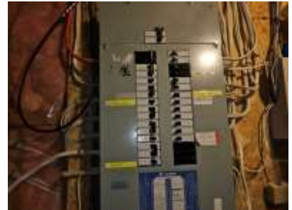
Pic. 39: 100 amp breaker panel
