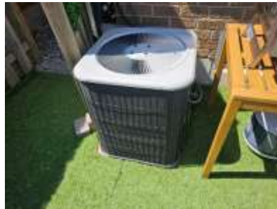
Pic. 8: AC unit 2017
