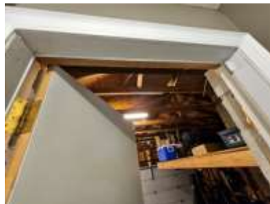
Pic. 11: Garage entry door has no auto closer and the wrong swing
