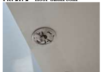
Pic. 24: Vendor to replace missing smoke / CO detector
