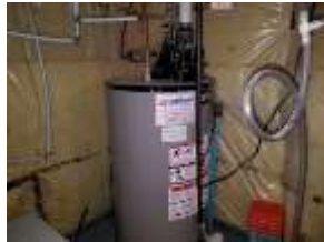
Pic. 30: Rental hot water tank
