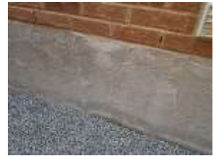
Pic. 8: Typical foundation crack
