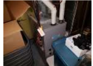
Pic. 28: High efficiency gas furnace
