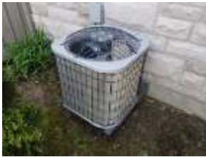
Pic. 5: AC unit
