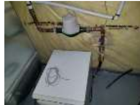
Pic. 31: Water main
