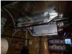
Pic. 29: HRV system – unplugged by owner
