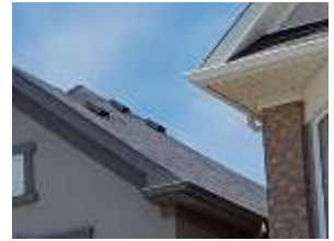
Pic. 4: Some shingle are cupping
