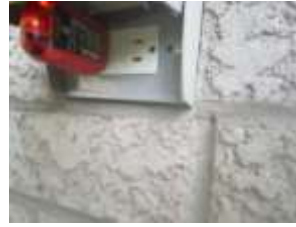
Image 3: Rear GFCI outlet won't trip needs replacement
