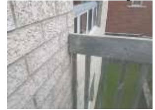
Image 24: Recommend securing the railing to the building
