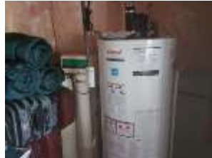
Image 30: Rental hot water tank
