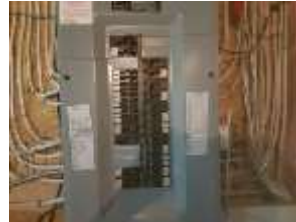
Image 31: 100 amp breaker panel with all copper wire
