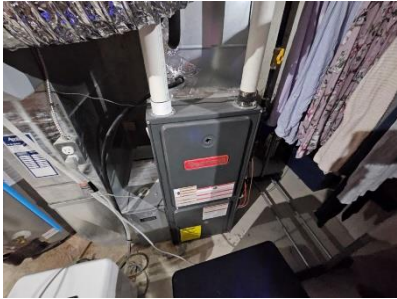
Pic. 34: Original gas furnace
