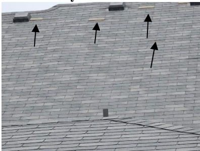
Pic. 7: Several missing shingle tabs on rear roof covering
