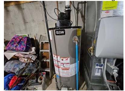
Pic. 33: Rental hot water tank
