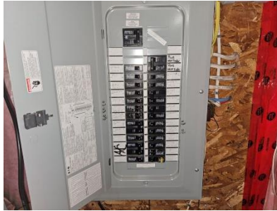
Pic. 35: 100 amp breaker panel
