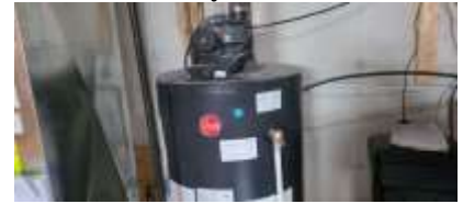
Pic. 30: Rental hot water tank 2012
