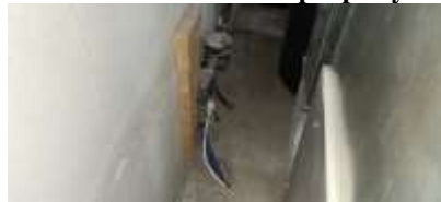
Pic. 32: Water main
