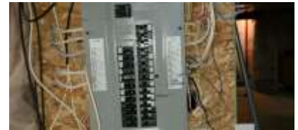
Pic. 33: 100-amp breaker panel
