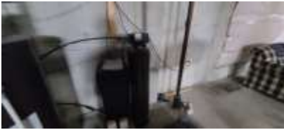
Pic. 28: Water softener
