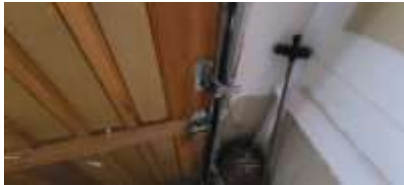
Pic. 7: Garage door latch cable disconnected
