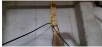
Pic. 29: Yellow wire is live and needs to be terminated properly
