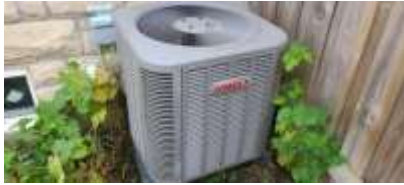
Pic. 4: AC unit 2012
