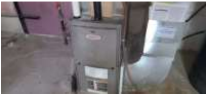
Pic. 31: Gas furnace 2012
