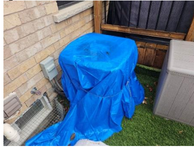
Pic. 32: AC Compressor 2022
