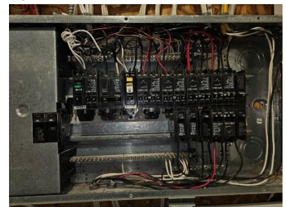
Pic. 30: 1200 amp breaker panel
