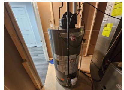
Pic. 27: Rental hot water tank 2021
