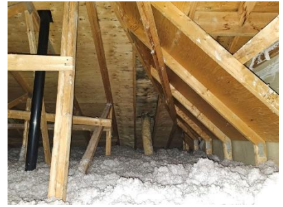
Pic. 6: Old moisture stains
