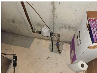
Pic. 29: Water main
