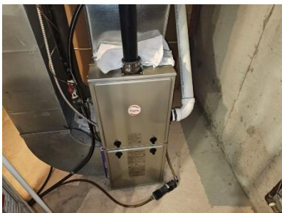
Pic. 28: Gas furnace 2022
