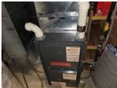
Pic. 29: Gas furnace 2024
