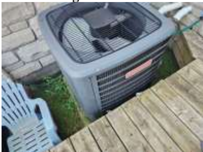
Pic. 7: AC compressor 2014
