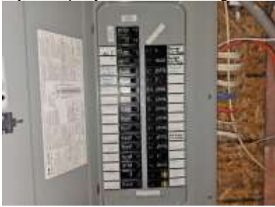
Pic. 31: 100 amp braker panel
