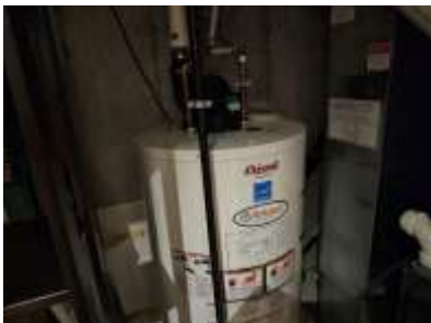
Pic. 28: Rental hot water tank 2021
