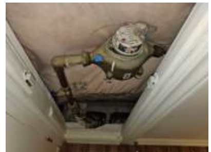
Pic. 30: Water main
