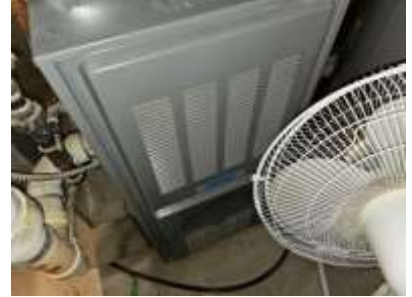
Pic. 32: Gas furnace 2008
