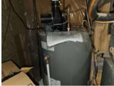
Hot water tank 2018
