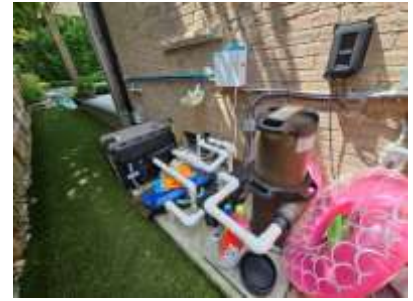
Pic. 3: Pool pump, filter and heater
