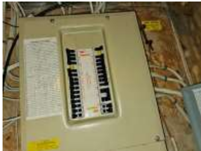
Pic. 34: 100 amp main electrical panel
