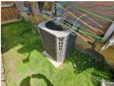
Pic. 7: AC unit
