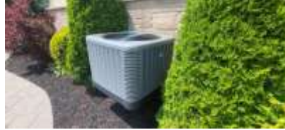
Pic. 5: AC unit 2018
