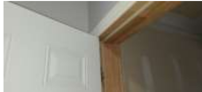
Pic. 11: Auto closer required for garage entry door
