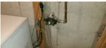
Pic. 37: Water main
