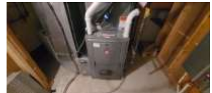
Pic. 36: Gas furnace 2018
