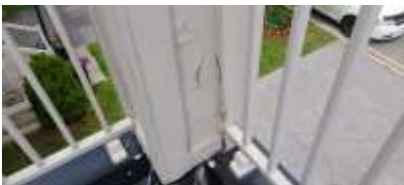
Pic. 13: Wood trim needs painting
