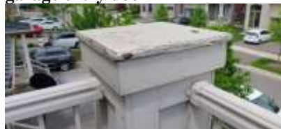
Pic. 14: Wood trim needs painting
