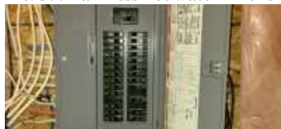
Pic. 38: 100-amp breaker panel
