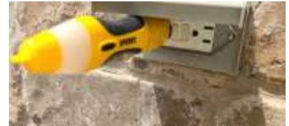
Pic. 9: Rear GFCI outlet defective
