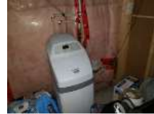
Pic. 35: Water softener – unplugged
