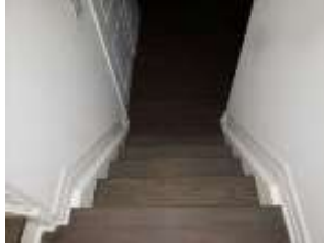
Pic. 29: Handrailing needed for basement stairwell
