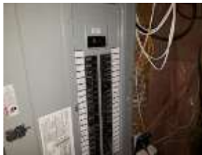
Pic. 37: 150 amp breaker panel
