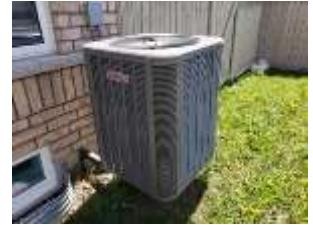
Pic. 4: AC unit 2014
