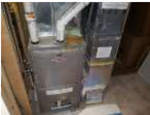
Pic. 36: +Gas furnace – recommend service and cleaning
