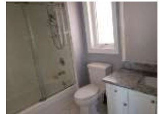
Pic. 19: 2 nd floor bath
