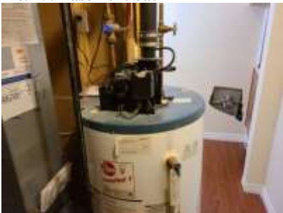
Pic. 28: Original rental hpt water tank
