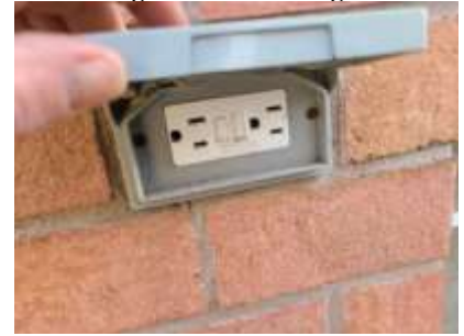
Pic. 6: Rear GFCI outlet needs replacement
