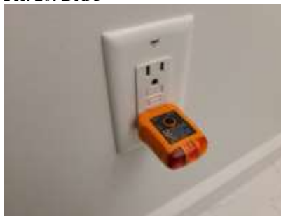
Pic. 23: Bathroom GFCI defective and needs replacement
