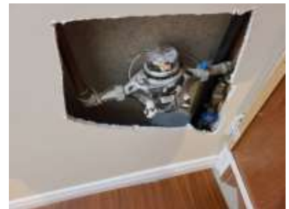
Pic. 27: Water main
