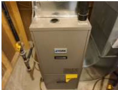
Pic. 29: Original gas furnace
