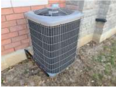
Pic. 4: Original AC unit
