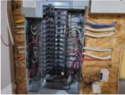
Pic. 31: 100 amp breaker panel
