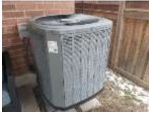
Pic. 5: AC unit 2006
