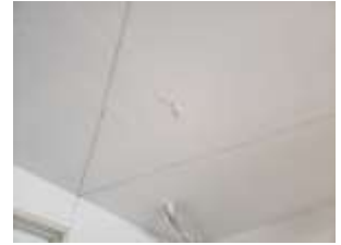
Pic. 8: Old water stain on ceiling all dry
