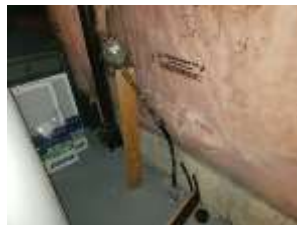
Pic. 38: Water main
