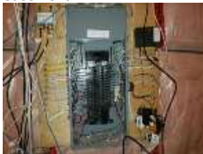
Pic. 41: 200 amp breaker panel
