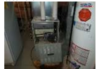
Pic. 40: Gas furnace 2010
