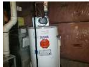
Pic. 39: Rental hot water tank
