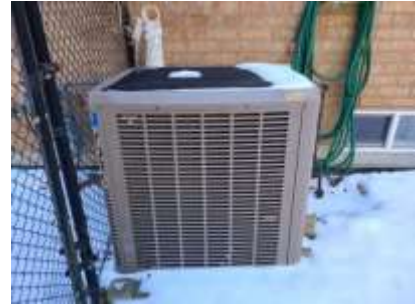
Pic. 3: AC unit 2009
