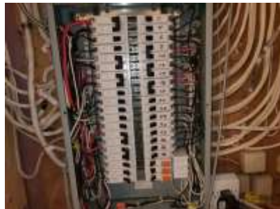
Pic. 41: 200 amp main breaker panel with all copper wire
