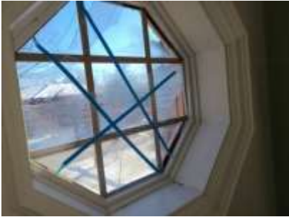
Pic. 19: Broken window
