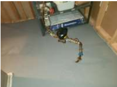
Pic. 40: Water main
