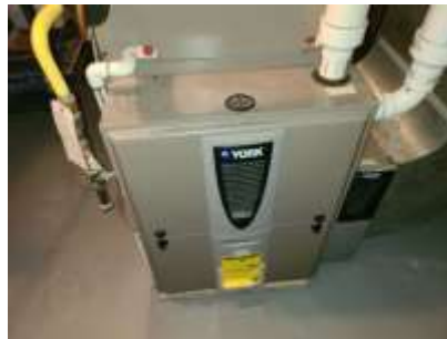
Pic. 38: Gas furnace 2010
