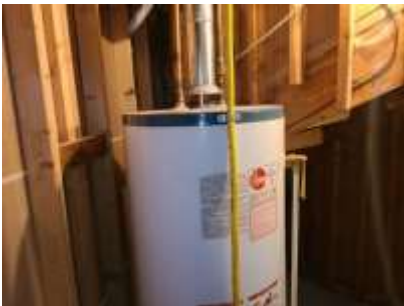
Pic. 37: Rental hot water tank
