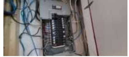
Pic. 30: 100 amp breaker panel
