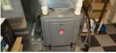
Pic. 25: Gas furnace 2021
