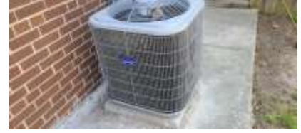
Pic. 3: AC unit 2021
