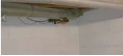
Pic. 28: Recommend capping or removing old oil tank fill / vent pipe
