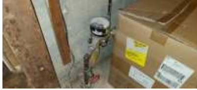
Pic. 29: Water main
