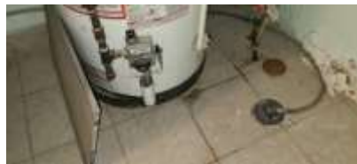
Pic. 20: TRP valve appears to have a small drip
