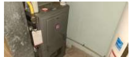
Pic. 21: Gas furnace 2017
