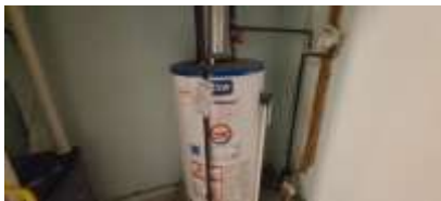
Pic. 19: Rental hot water tank
