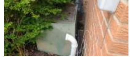
Pic. 24: Aged AC compressor
