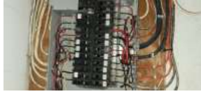
Pic. 23: 100 amp breaker panel with 60% copper wire and 40% aluminum
