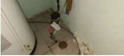
Pic. 22: Water main
