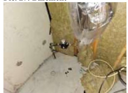
Pic. 30: Water main
