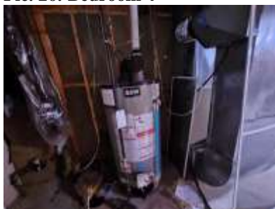
Pic. 29: Rental hot water tank
