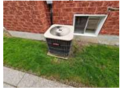
Pic. 6: Original AC unit
