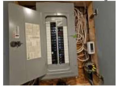
Pic. 33: 100 amp breaker panel
