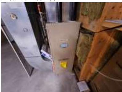
Pic. 28: Original gas furnace
