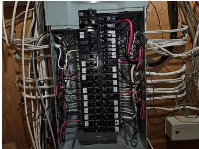
Pic. 34: 100 amp breaker panel
