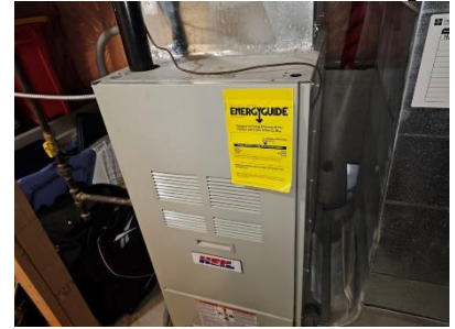
Pic. 33: Gas furnace 2001
