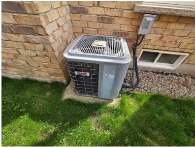
Pic. 4: AC unit 2001
