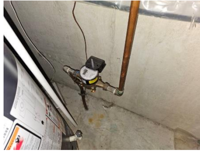
Pic. 32: Water main
