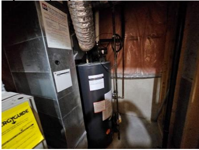
Pic. 31: Rental hot water tank 2012
