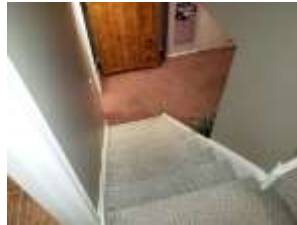
Pic. 30: Handrail needed for basement stairwell
