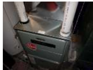
Pic. 39: Gas furnace 2009
