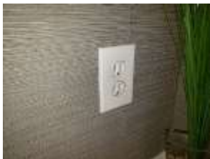
Pic. 37: No GFCI in basement bath
