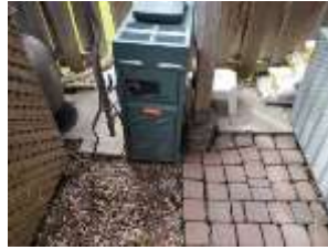
Pic. 6: Pool heater
