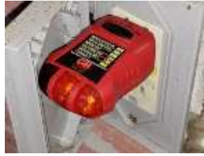
Pic. 2: Exterior GFCI needs replacement
