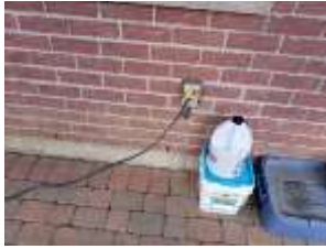
Pic. 5: Improper extension cord wiring for pool equipment
