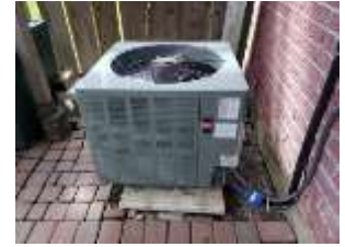
Pic. 8: AC unit 2008
