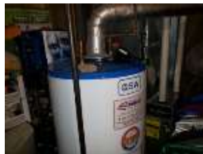
Pic. 38: Rental hot water tank 2008
