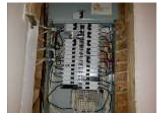
Pic. 40: 100 amp breaker panel
