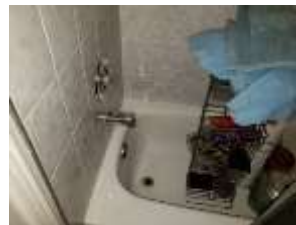
Pic. 19: 2 nd floor bath
