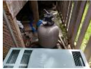
Pic. 7: Pool equipment
