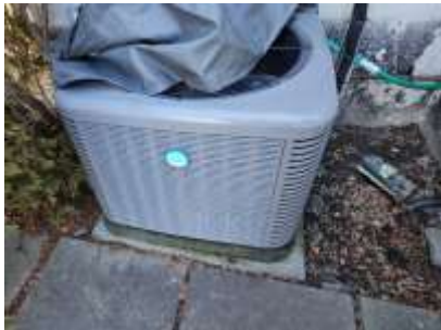
Pic. 7: AC unit 2016
