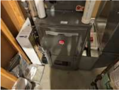
Pic. 31: Gas furnace 2016
