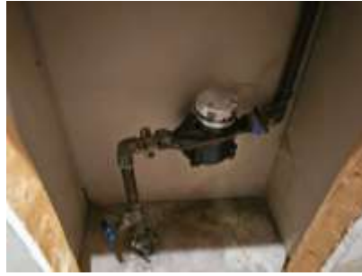
Pic. 32: Water main
