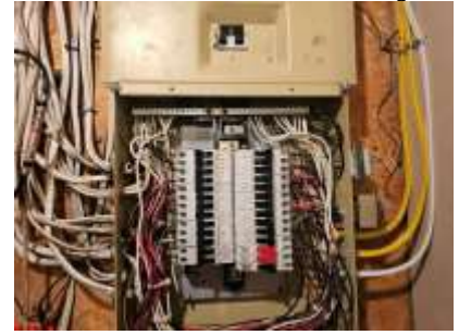
Pic. 33: 100a amp breaker panel
