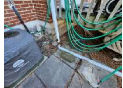
Pic. 6: Downspout extension needs to be connected
