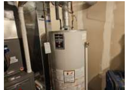
Pic. 30: Hot water tank 2016
