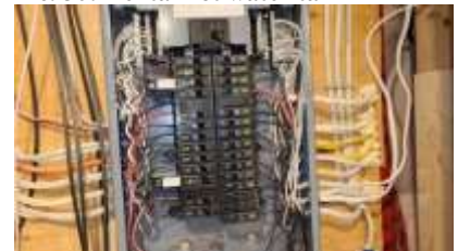
Pic. 33: 100 amp breaker panel
