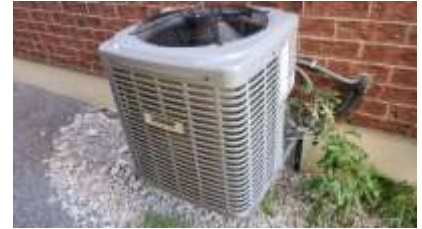
Pic. 3: AC unit 2013
