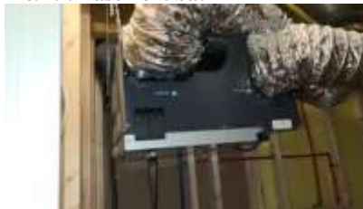
Pic. 32: HRV system
