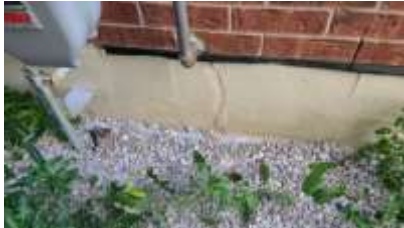
Pic. 4: Typical foundation crack
