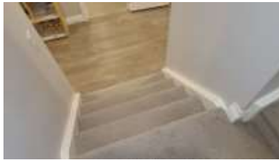
Pic. 26: Hand railings needed for basement stairwell
