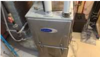
Pic. 31: Original gas furnace
