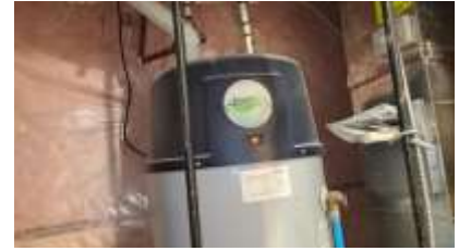
Pic. 30: Rental hot water tank
